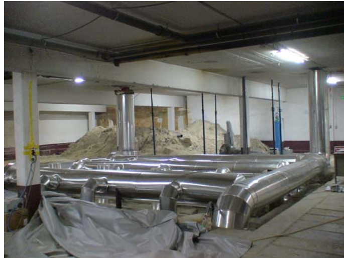
Fig 3bis. Pipe network on the polluted area
