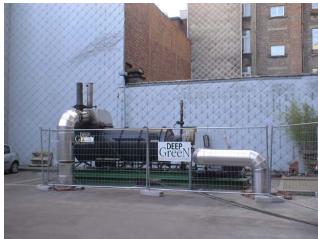
Fig4. Thermal oxidizer installed outside, on the ground floor, just above the polluted area
